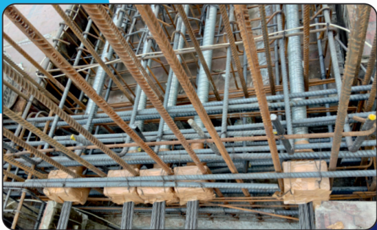
Live End of Bonded PT System
