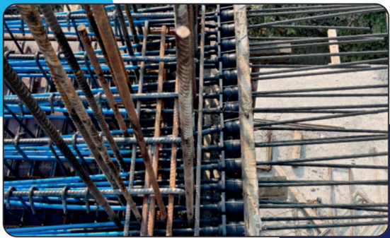
Live End of Unbonded PT System
